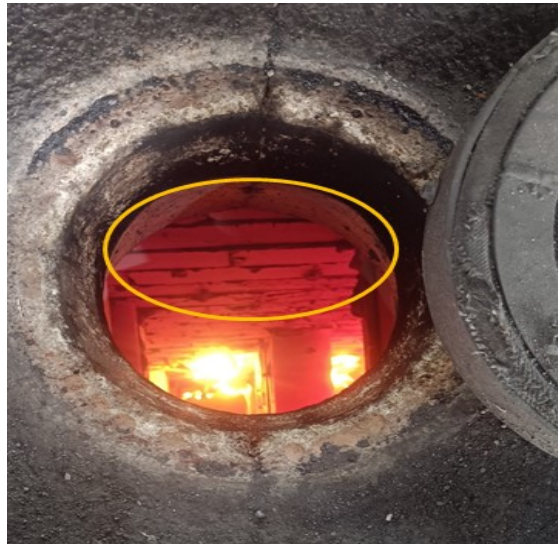
Figure 6. Flue cavity showing deposition of fuel at the bottom.
